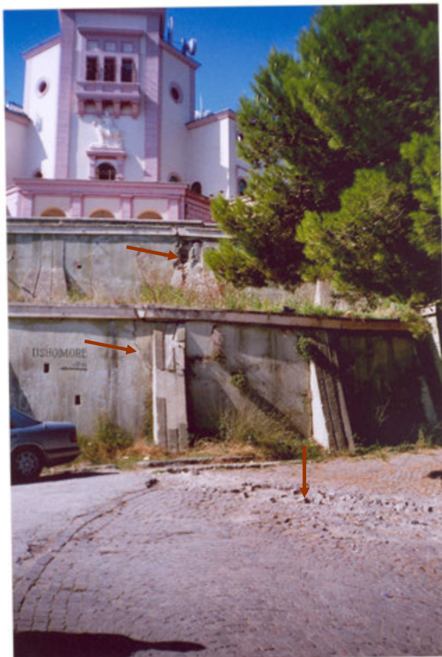
Cracks in the villa walls and transversaly of the road
