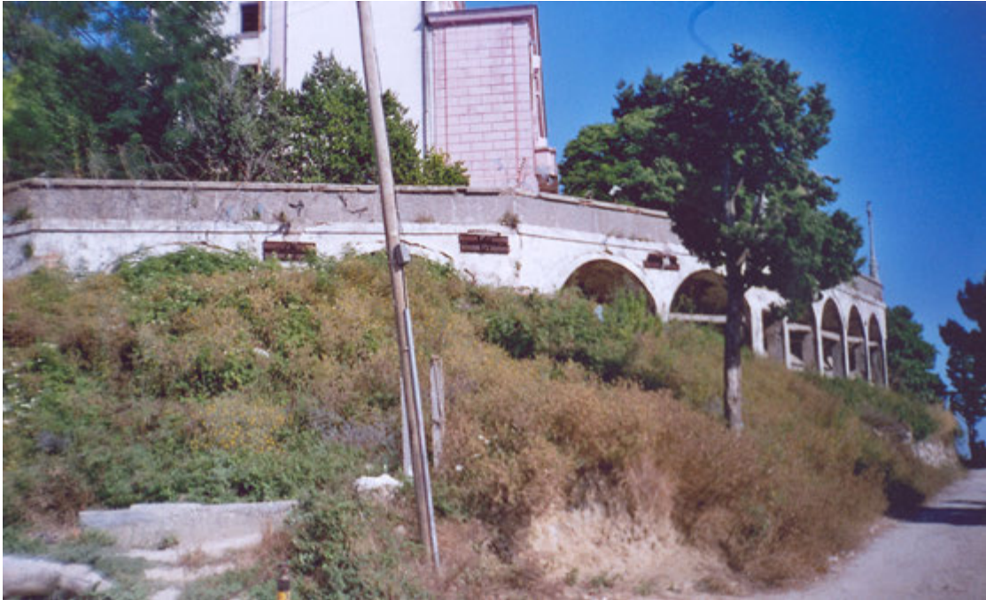
Subsidence of the villa wall, caused by landslide
