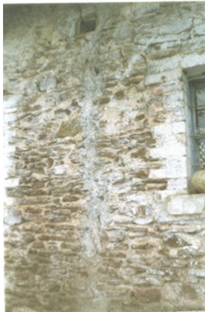
Cracks of the village houses walls
